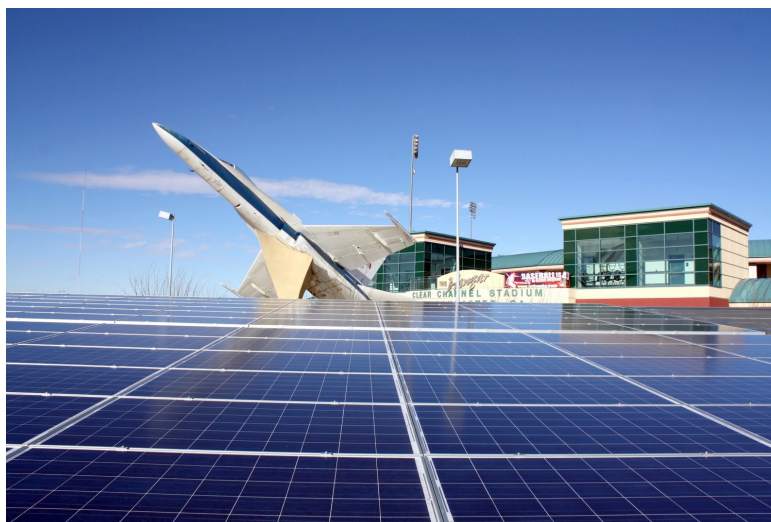
Parking lot canopy solar array at Lancaster Jethawks stadium. Credit: Todd Woody
