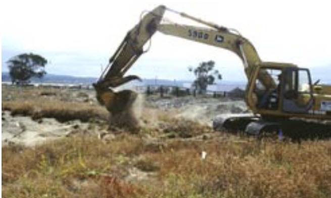
Using heavy equipment to remove invasive plants from a Bureau of Land Management Endangered Plant Protection Area. This work was organized using a cooperative agreement between Redwood Community Action Agency and the BLM. RCAA contracted with a local private heavy equipment operator for project implementation. Photo credit: Andrea Pickart, USFWS.
