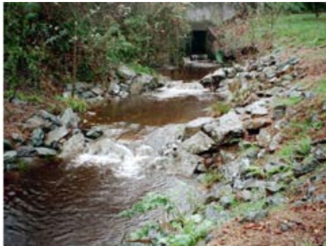
Part of a culvert modification project on the main stem of Widow White Creek. Shown is the installation of three rock weirs to create jump pools that reduce the overall jump height from one 3-foot jump at the culvert outlet to three 1-foot jumps. Funding was provided by grants from the Department of Water Resources – Urban Streams Restoration Program. Project partners included Loring Swanlund of Ocean West Senior Village and the McKinleyville Community Services District. Photo credit: Don Allan, Natural Resources Services, RCAA.
