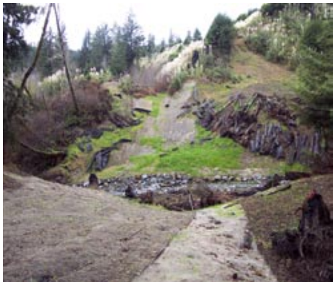
A sequence showing the excavation of an old abandoned railroad crossing with a 80-year old 36-inch redwood box culvert that was threatening to fail. Two excavators removed over 10,000 cubic yards of unstable soil materials and loaded them into dump trucks. Channel side slopes were excavated back to a stable, low gradient angle and protected with mulch, jute netting, and plantings. The channel bottom was rock armored. This restoration project and the one pictured on page 32 were implemented on Simpson Resource Company property in the Little River watershed. In both cases, Pacific Watershed Associates worked with the nonprofit organization Pacific Coast Fish, Wildlife, and Wetlands Restoration Association on project planning, management, and reporting; local heavy equipment operators were employed for project implementation. The projects were funded by the California Department of Fish and Game, with additional partial match funding from Simpson Resource Company. Photo credit: Pacific Watershed Associates and the California Department of Fish and Game.
