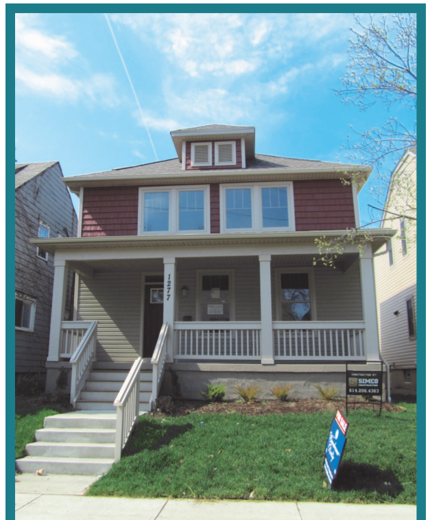
A federally-funded Neighborhood Stabilization Program (NSP) home renovation on North 5th Street in Weinland Park
