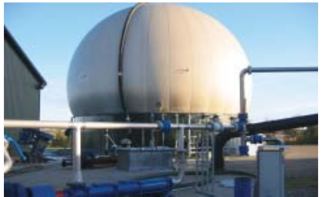
D.12 Hashøj biogas storage tank
