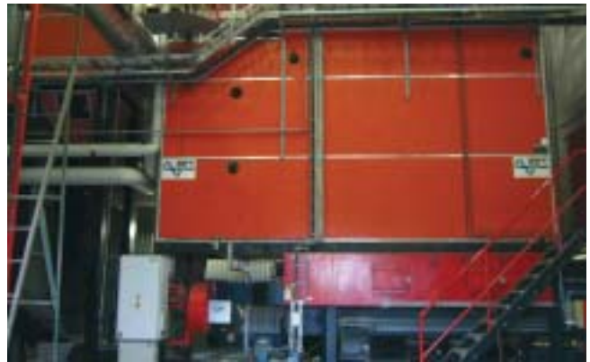
S.2 Farmarenergi: heating plant boiler
