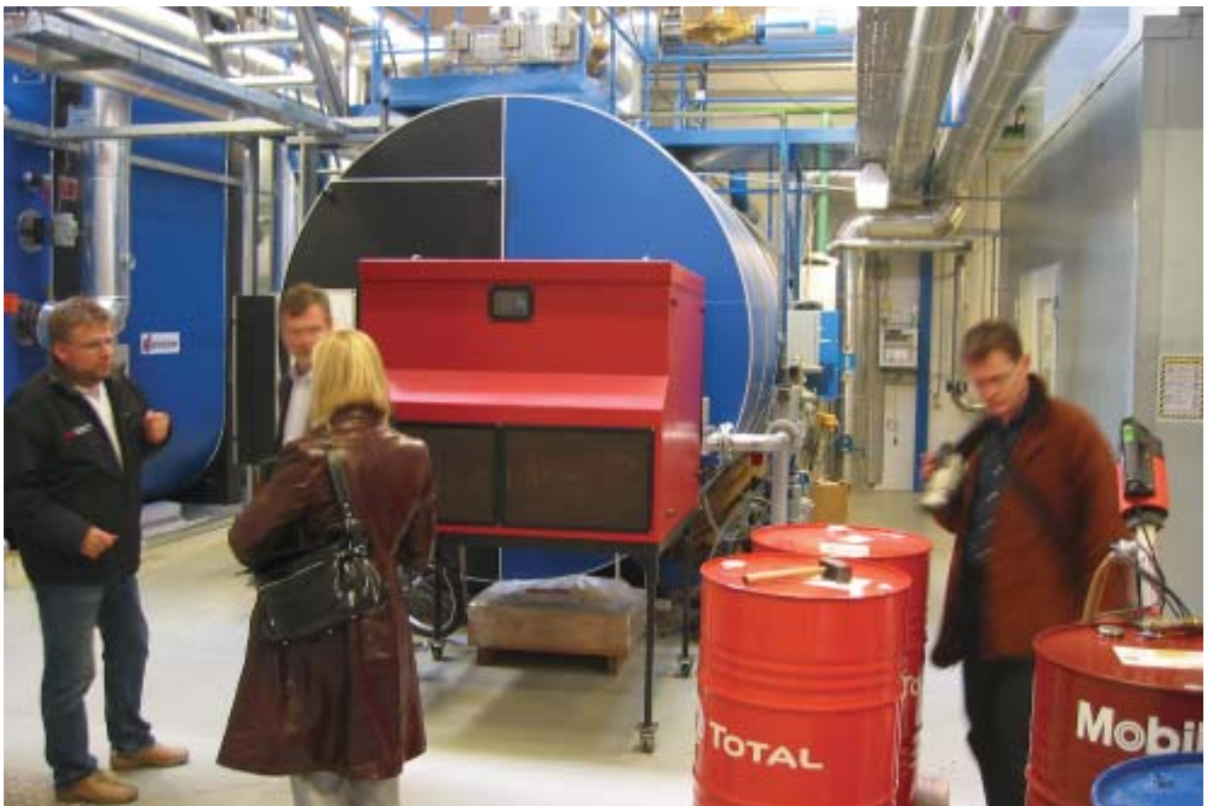
D.16 Hashøj CHP station internals
