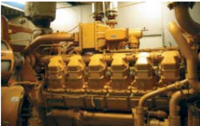
D.11 Hashøj biogas CHP engine
