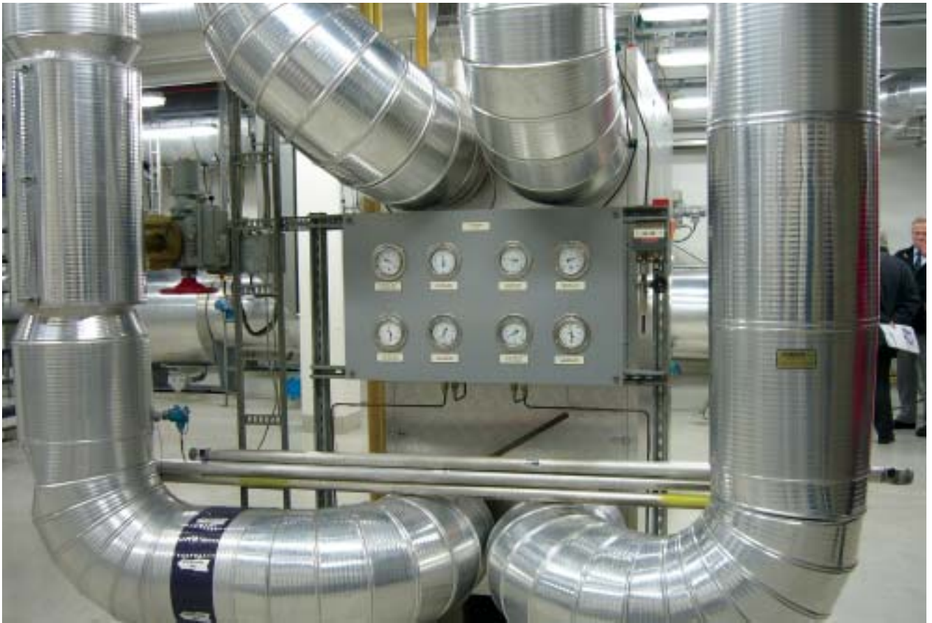
D.10 VEKS heat exchanger display
