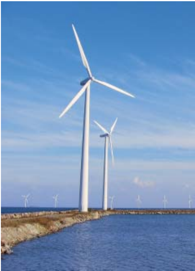
D.4 Lynetten wind farm with Middelgrunden in distance
