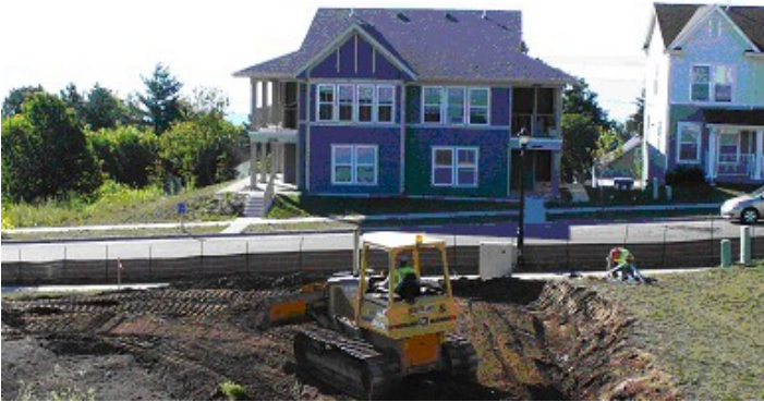
Harbor Highlands – Phase I – “A Village with a View” - 44 on-site units including 11 public housing units, 7 of which are occupied by HOPE VI residents
