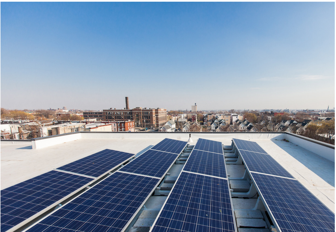
Above: Solar panels at Paseo Verde and view of Philadelphia
